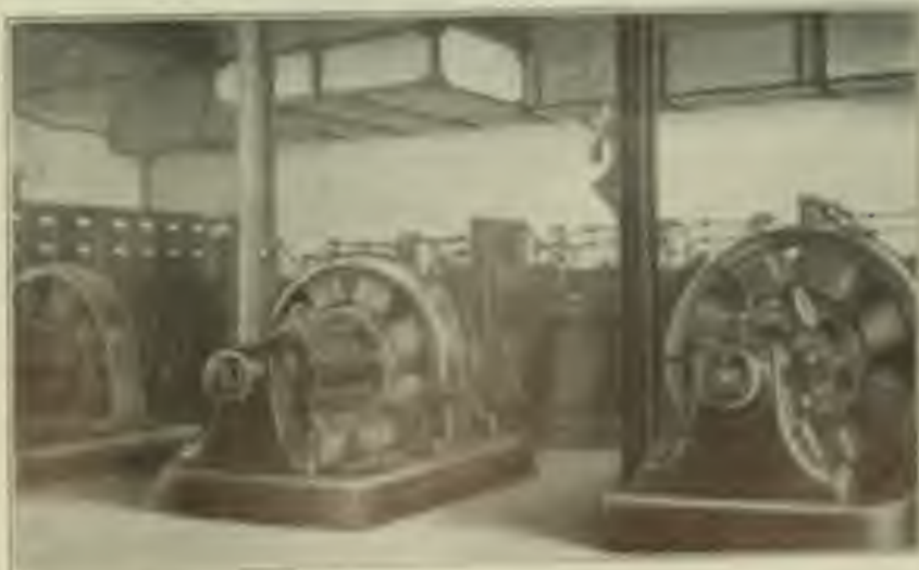
FIG. 6 Auxiliary connections in generator
